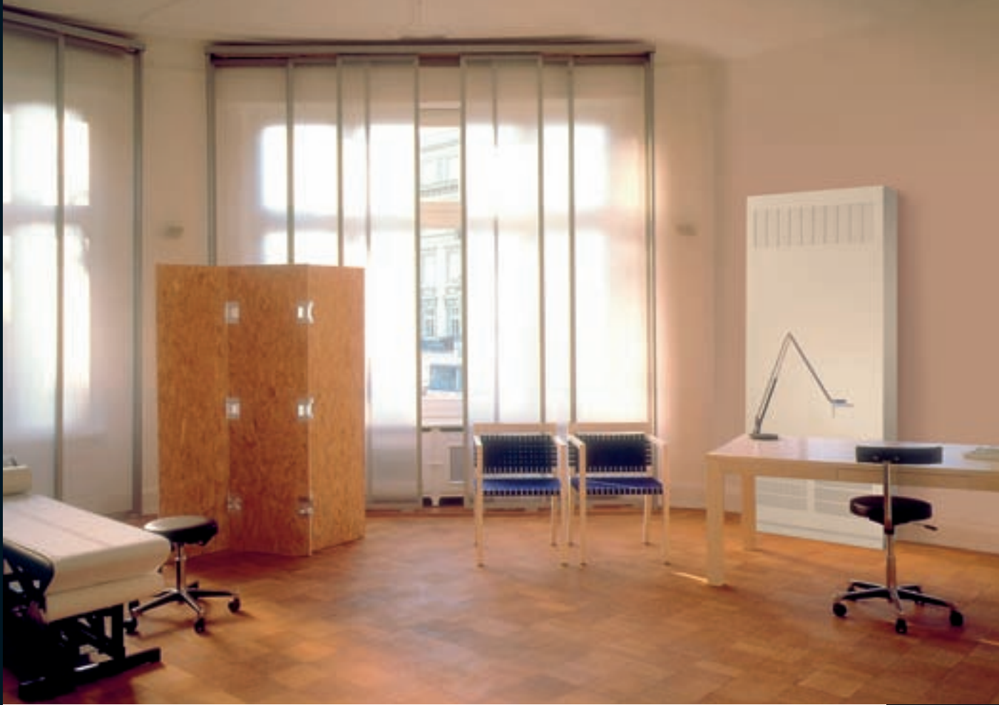
The Zehnder COS Cooling Duct in a medical practice.
